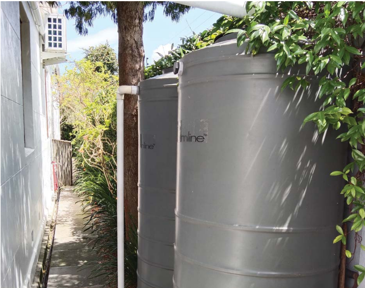
Figure 17: Rainwater harvesting tanks efficiently collect rainwater for garden irrigation.
